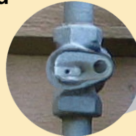
Closed gas meter valve
